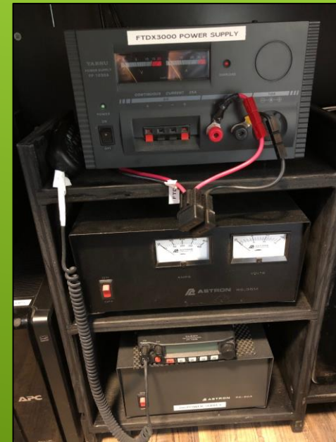
AC4G's Power Cabinet w/ 2m VHF Yaesu Rig (bottom)
